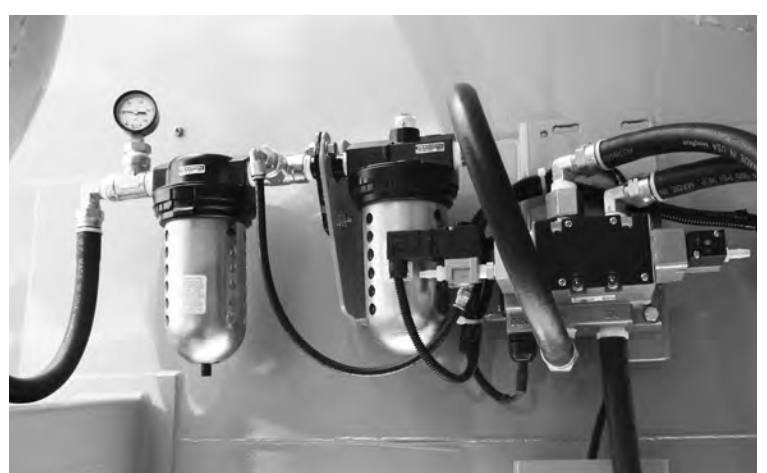
USA steel cylinder configuration Clam Gate
